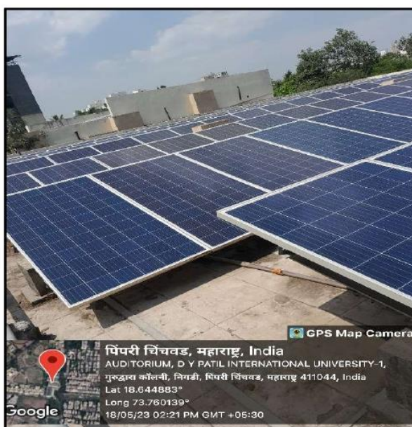
Photograph of Roof Top Solar PV Plant:
