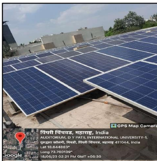
Photograph of Roof Top Solar PV Plant:
